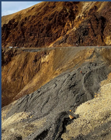
▲ The landslide at Pretty Rocks in Denali National Park has caused regular road cancellations and hindered access to the park. (photo: National Park Service)
